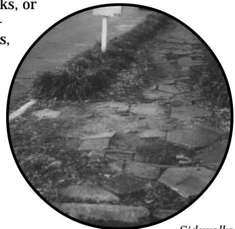
Sidewalks with cracked, uneven pavement and no ramp make it difficult for strollers and wheelchairs to cross.
